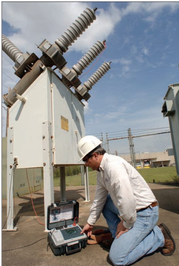
The MIT1020 in use at an industrial complex substation
